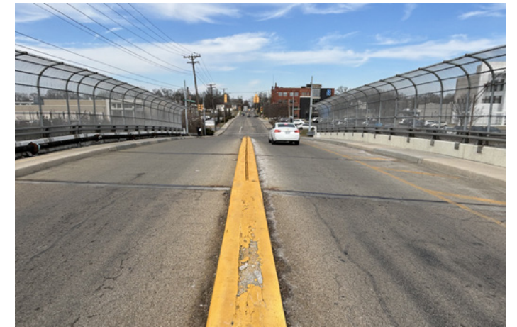
Section Avenue bridge has narrow sidewalks and wide car lanes, without bicycle treatments.
