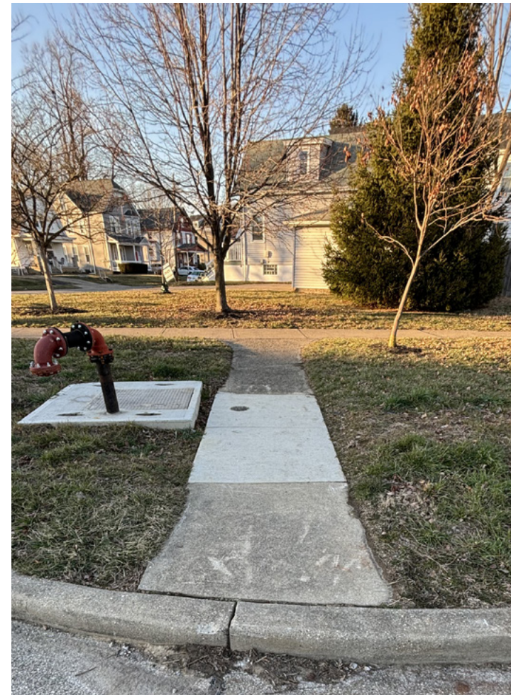
Missing ADA curb ramp to the sidewalk.
